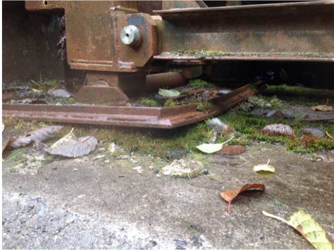
left upstream bearing
